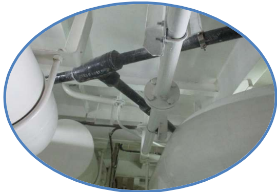
Seawater Cooling Piping
