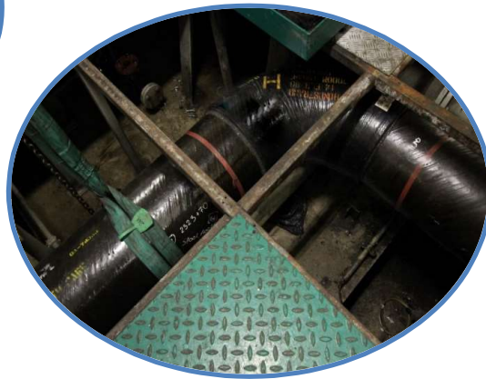
Ballast Water Piping
